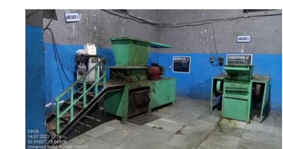
Two Shredders of total capacity 550 kg/hr at CBWTF
