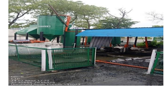
View of ETP at CBWTF
