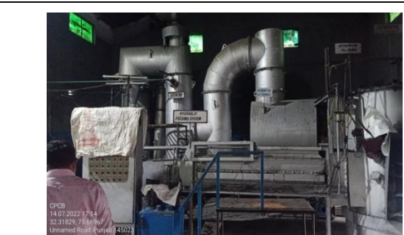
Incinerator of capacity 150 kg/hr at CBWTF
